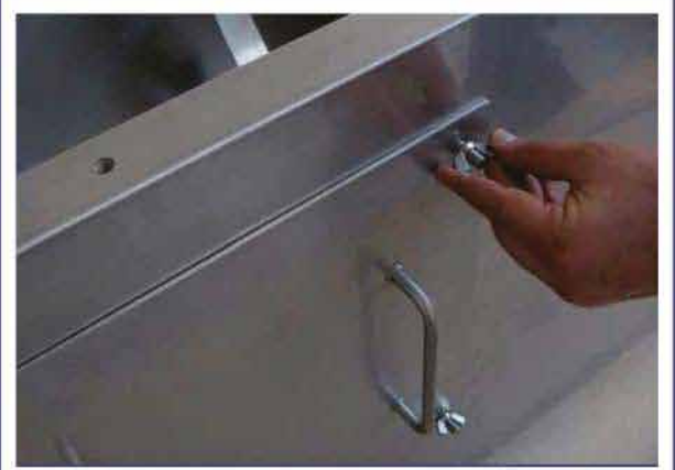
DOOR FOR INSPECTION
